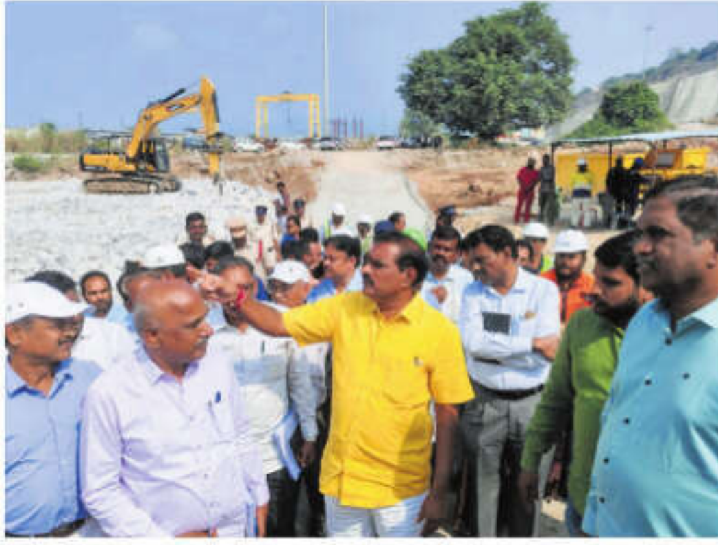
Water Resources Minister Nimmala Ramanaidu inspects Gap-1 and Gap-2 works of the Polavaram Project during his field visit on Thursday | EXPRESS
