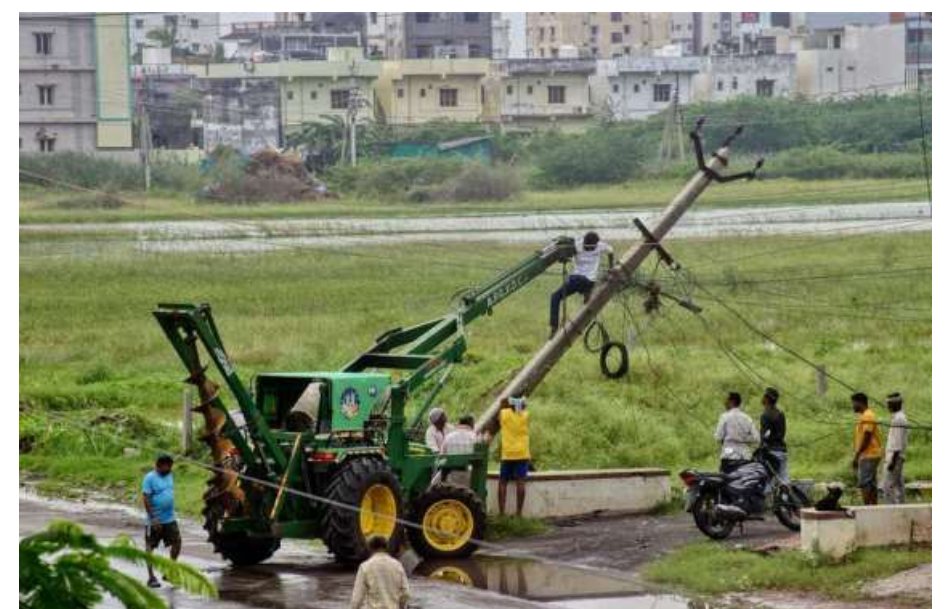
Officials repairing an electric pole uprooted by strong winds triggered by Cyclone Montha in Ongole on Wednesday. KOMMURI SRINIVAS
