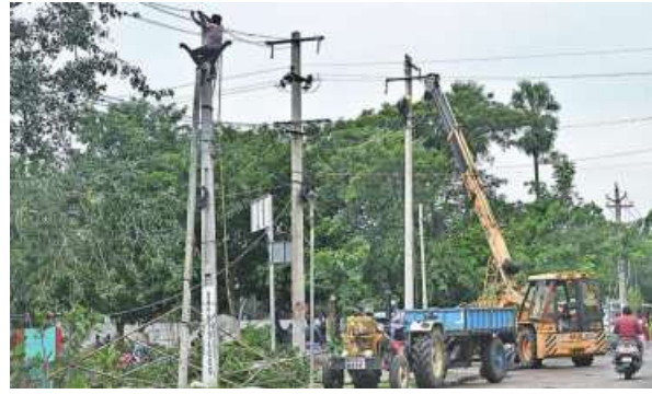
Electricity department employees carrying out repairs to damaged lines, in Machilipatnam on Wednesday. K.V.S. GIRI
